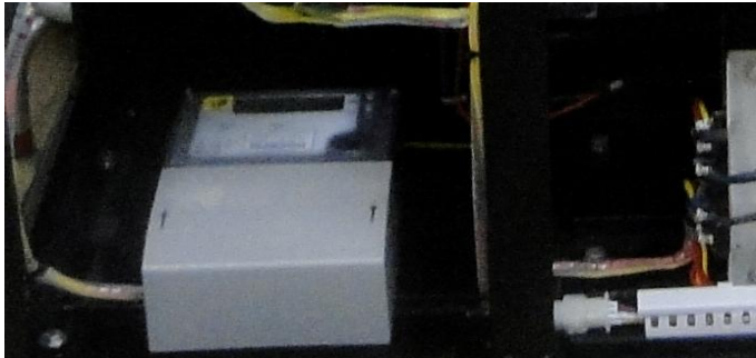
PQMS meter mounted inside 3 Phase SCR V PropSava
