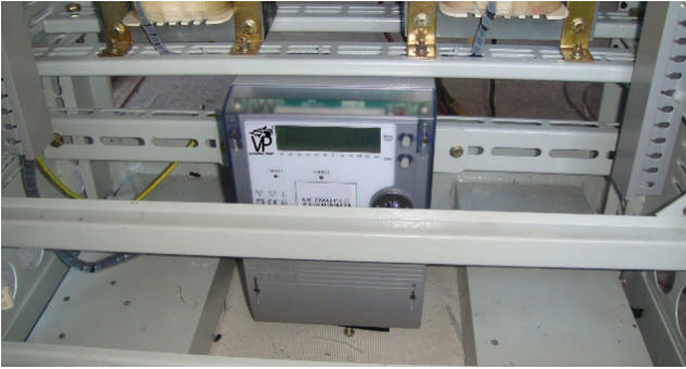
PQMS meter mounted inside 3 Phase SCR PropSava
