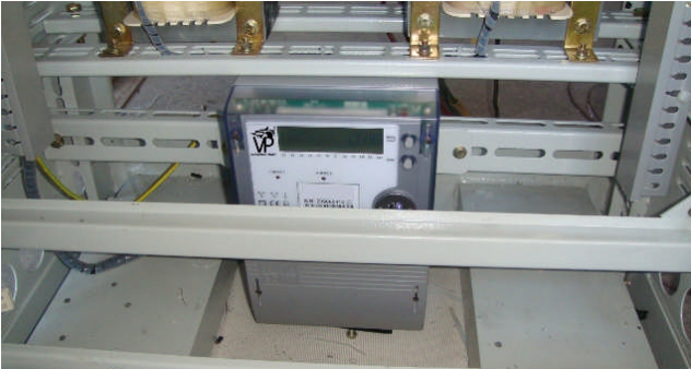
PQMS meter mounted inside 3 Phase SCR PropSava
